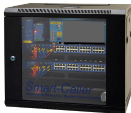
Fig. 2 128-INPUT NODE READY FOR SHIPMENT
